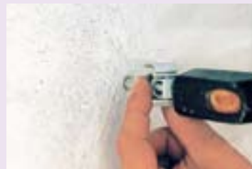
Strike conduit support
