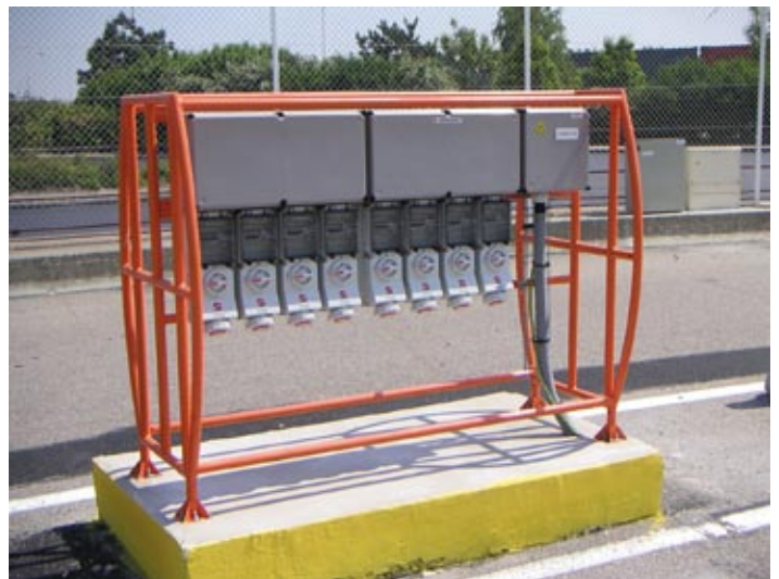
Container Terminal, Le Havre – France
